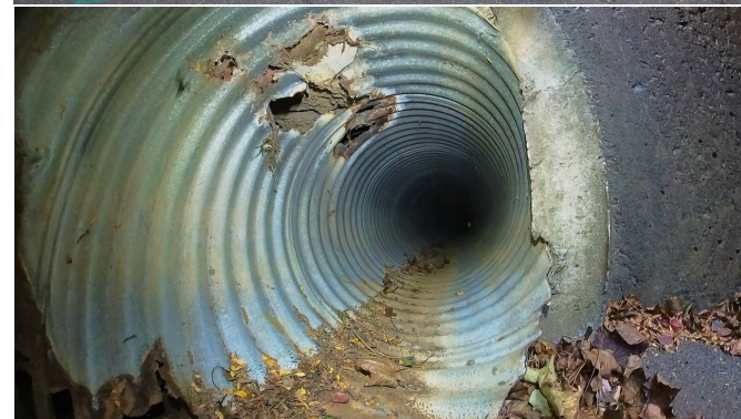
Failing Pipe on Danberry Drive
